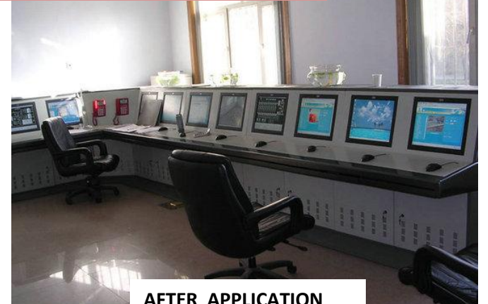
Control Centre Room (south)
